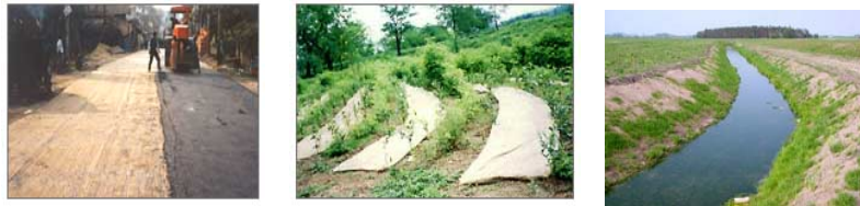
Geo-jute applications for road construction, vegetation and soil saving/erosion control activities respectively.
